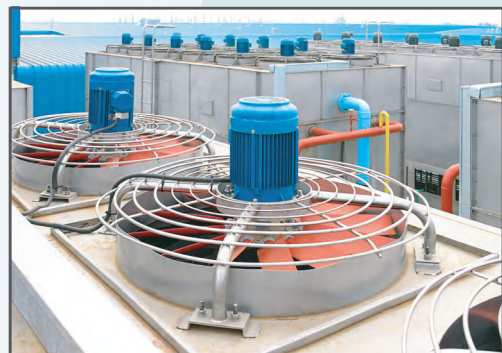
Fan and water pump
